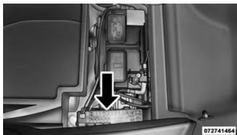
Rear Power Distribution Center
